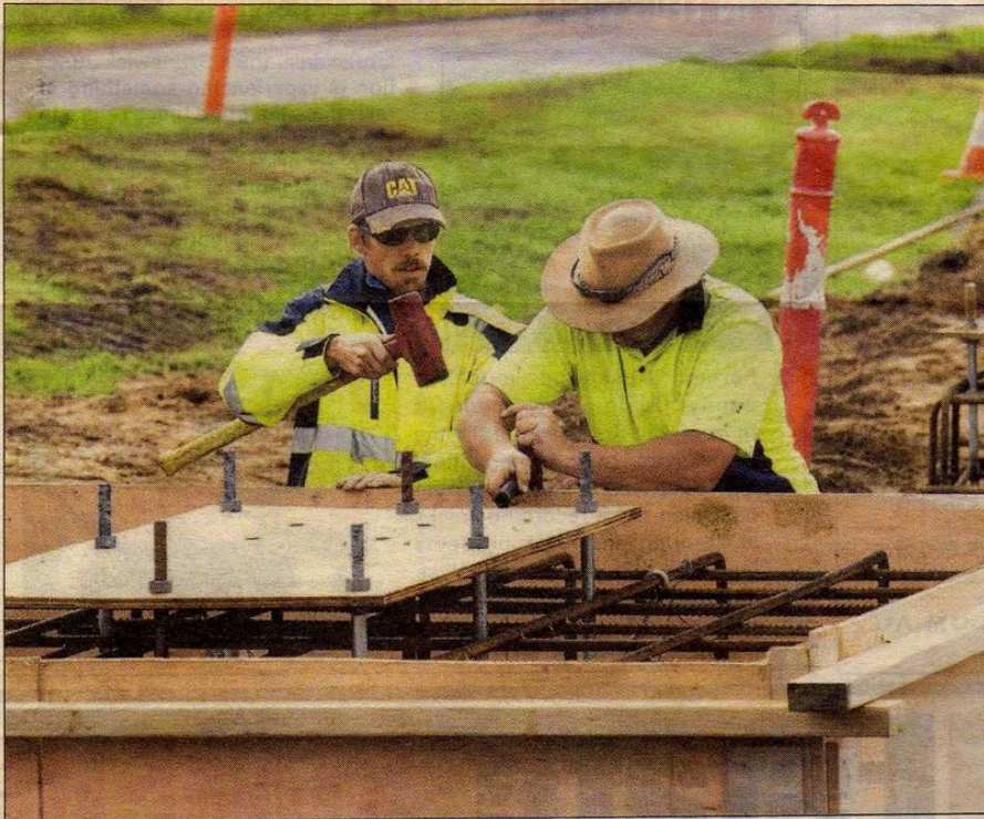
Workers Mark Burchell and Tory Baxter are busy constructing the base for Bunbury's new northern entry statement. PICTURE: HENRY LAM
